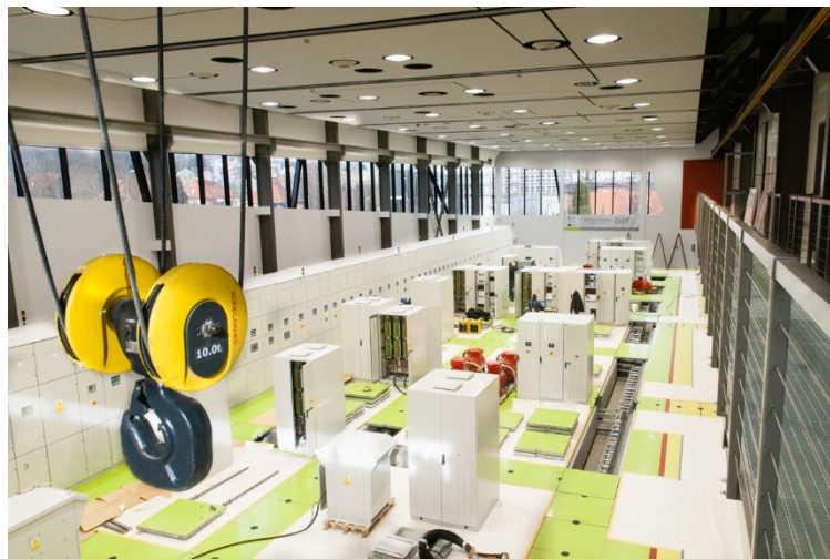
Figure 1: The main space of LINTE 2 Lab - an array of functional units and the main electrical switchgear (photograph by Piotr Niklas).
